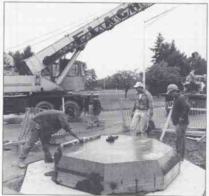
The 12,000 pound base is set into place by Flach Crane & Rigging Co.
